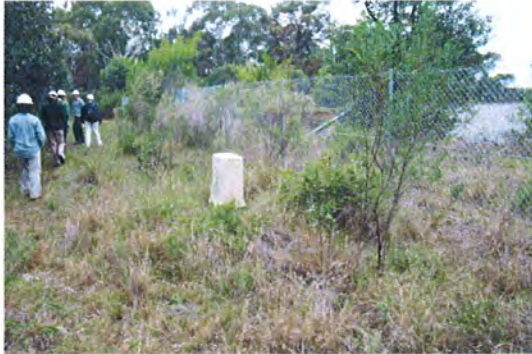
Figure 5.1 Electrical infrastructure within the woodland area.
