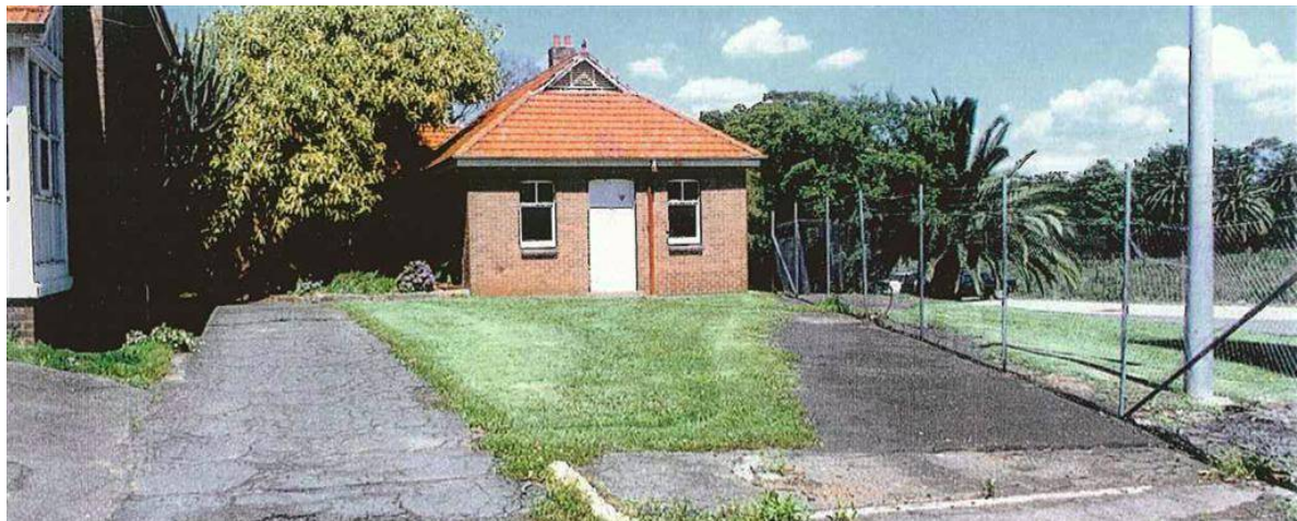
Figure 145 Eastern façade of Building C. Note the enclosed verandah of Building B to the left. 1995 Source: Conservation Study, Playfair Memorial Fountain Homebush, 1995
