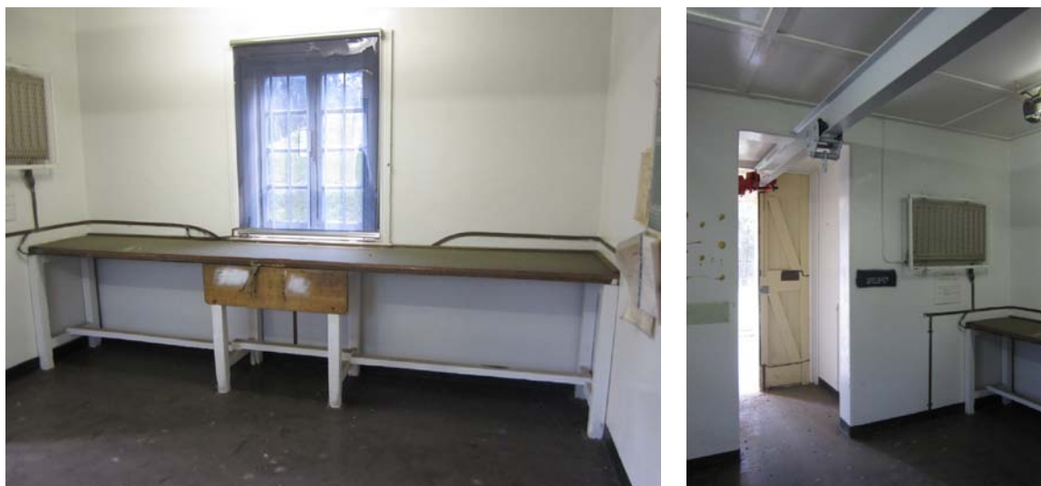
Figure 3-60 Earthing strips associated with work areas and a gantry in Building 155 (Source: Tanner Architects).
