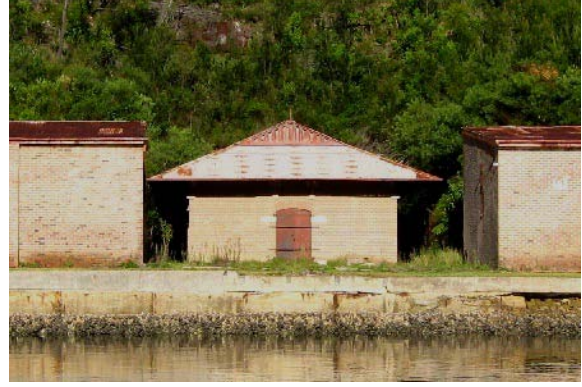
Figure 4-2 Bantry Bay was built as the primary public magazine in NSW. It occupies the foreshores of a harbour inlet (Source: Tony Brassil).
