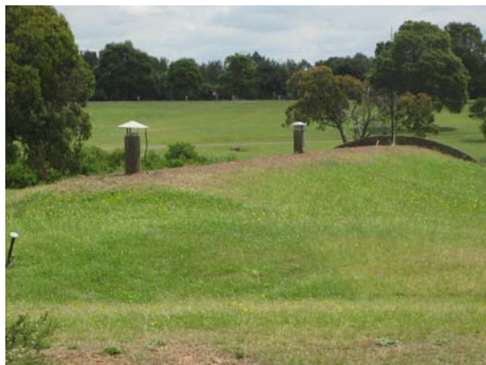
Figure 3-70 The “roofs” and vents of the storehouses contribute to the character of this section of the Armament Depot (Source: Tanner Architects).
